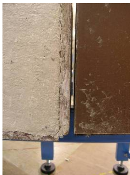
Figure 1-44. Gap between Scattering Box Concrete Blocks.
