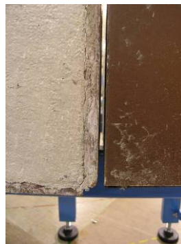
Figure 1-47. Gap between Scattering Box Concrete Blocks.
